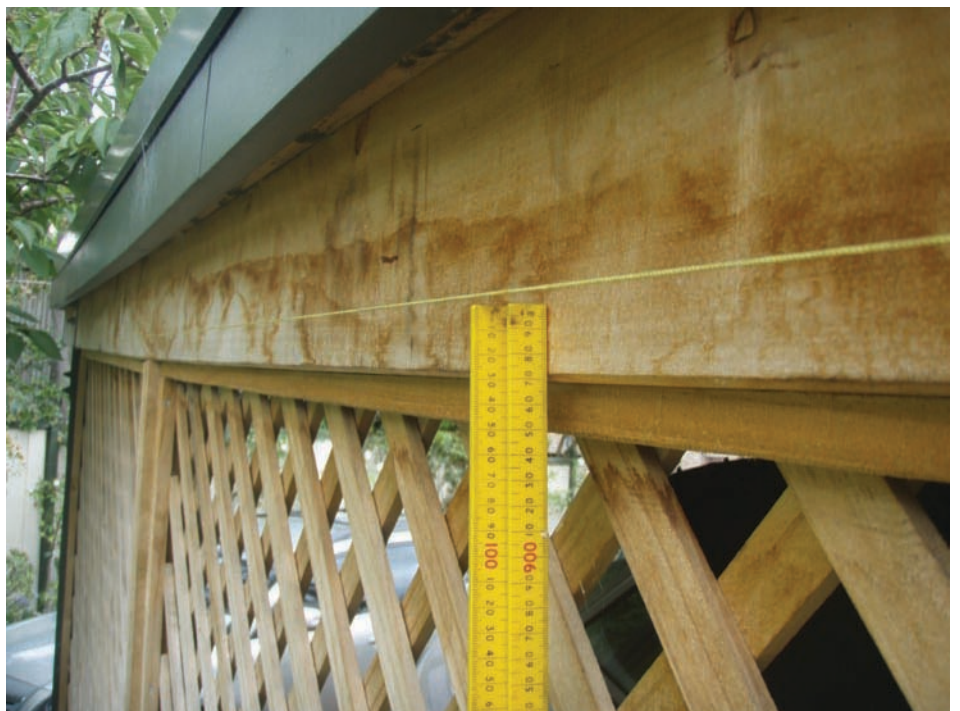
The 35 mm sag in the beam, the fascia and, of course, the roof. Note the camouflage attempt of trellis for a future climbing rose.
