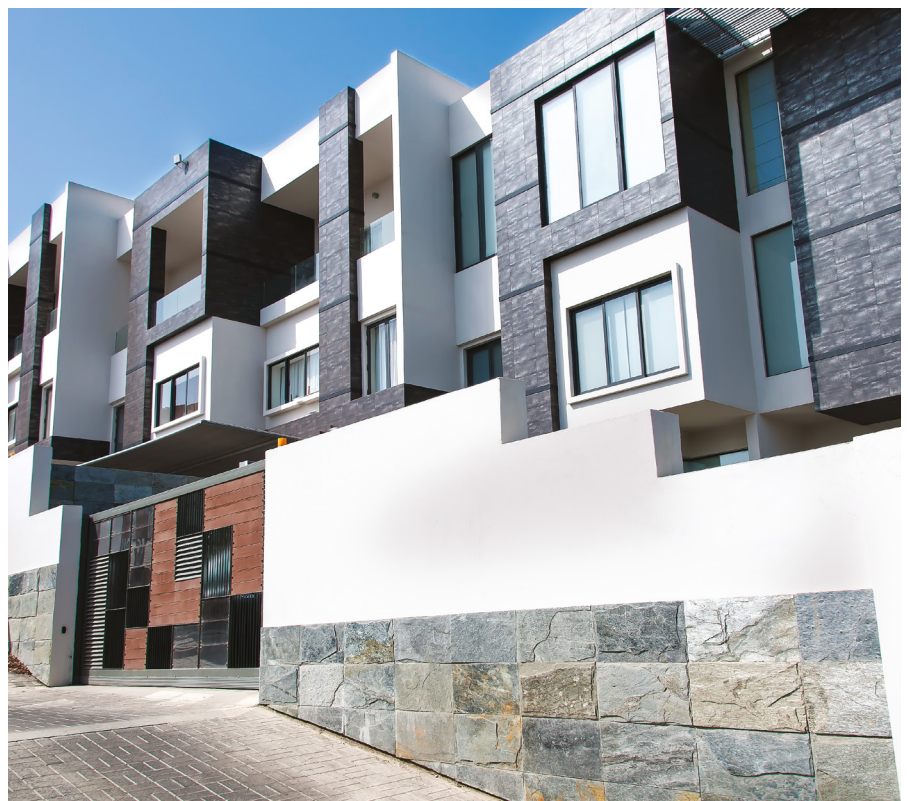
Certain design features can increase maintenance requirements. In this example, the boxed windows will need more attention to ensure weathertightness.
