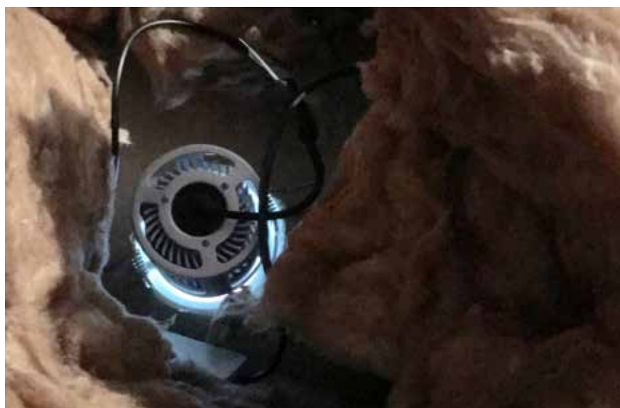
The gap around a downlight in the Titirangi house is clearly visible.
