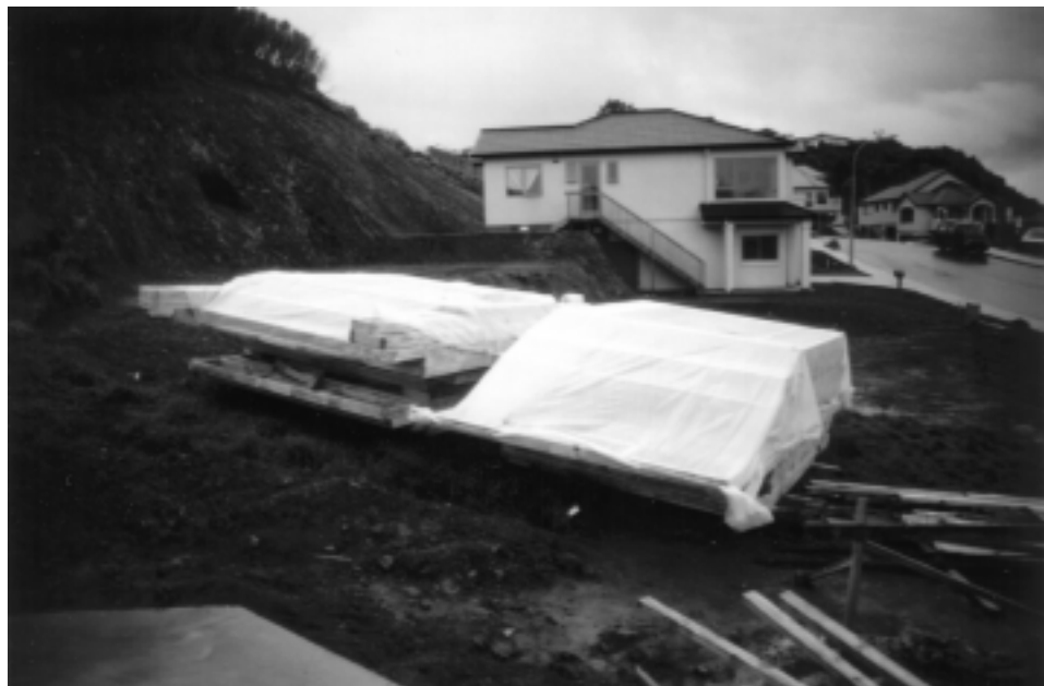
Poorly protected frames.
