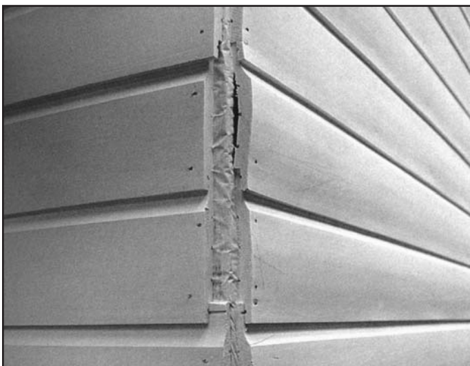
Consequences of rusticated weatherboards that were installed without an expansion gap. (Note the incorrect double nailing.)
