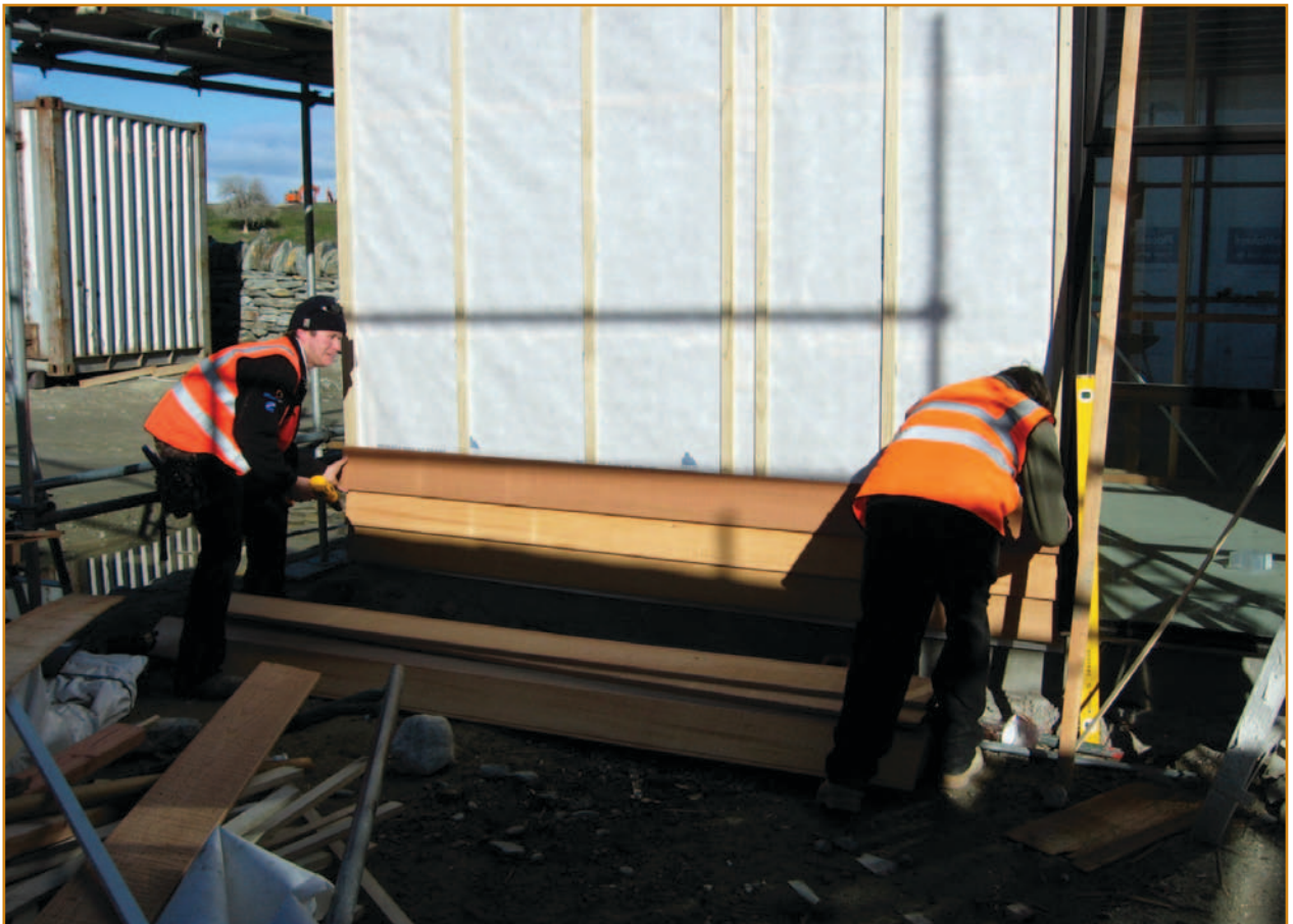
Typical example of timber weatherboards being installed over an E2/AS1 20 mm cavity.
