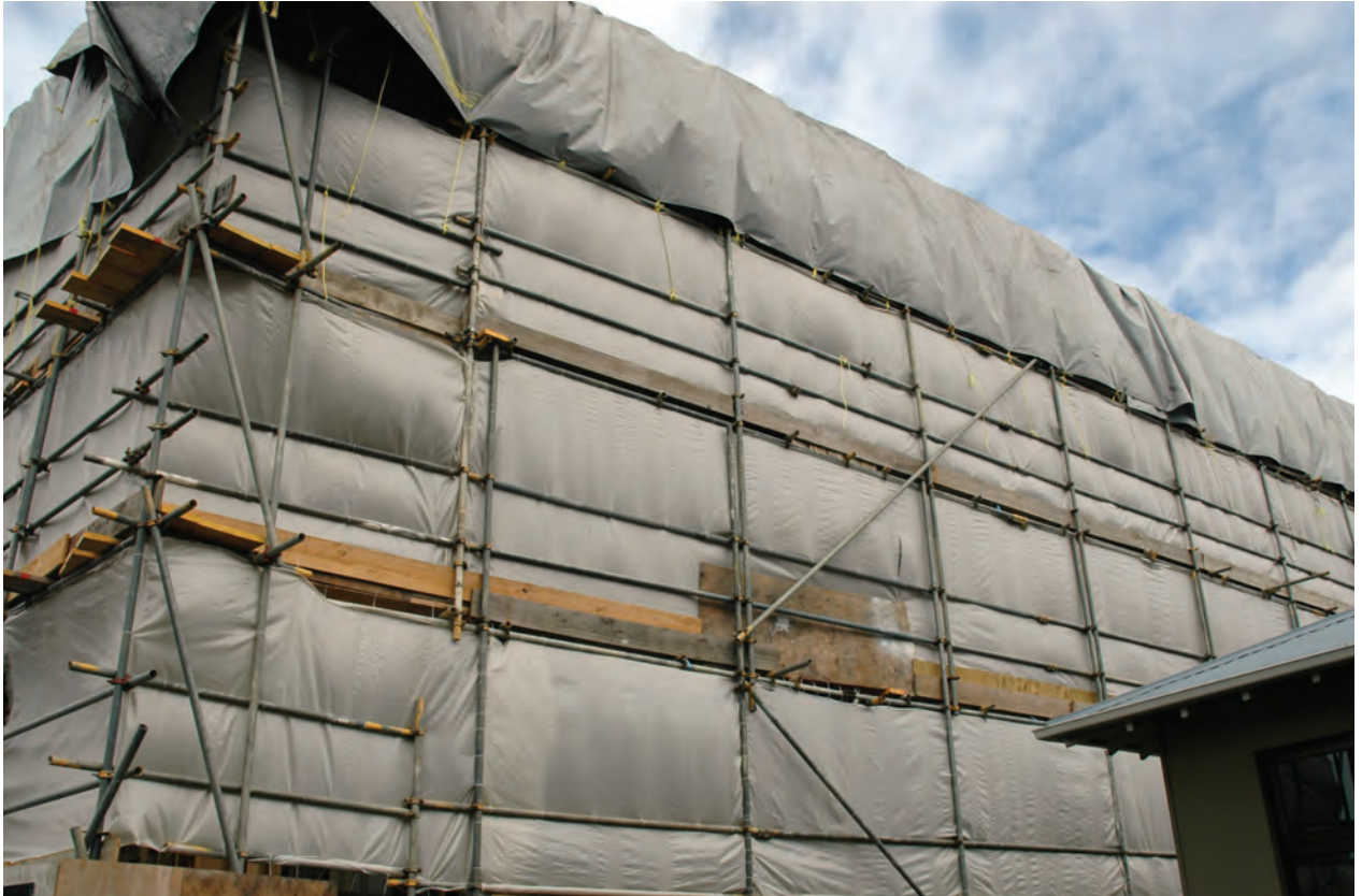
Figure 3 Full cladding replacement allows all faults and decay to be found and exposed timber to be treated.
