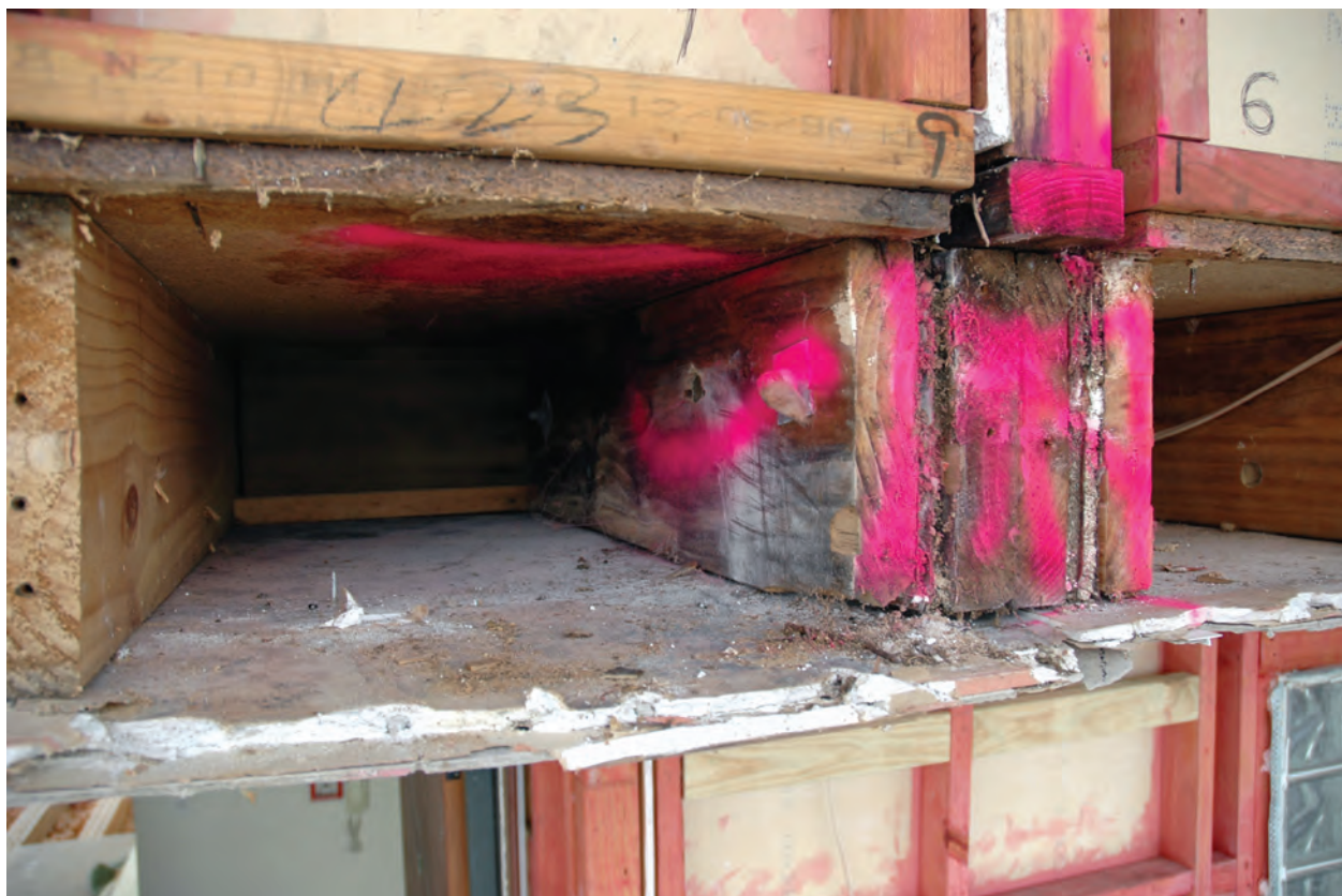
Figure 1 Rot in the ends of intermediate floor joists, with deterioration also visible in the flooring.
