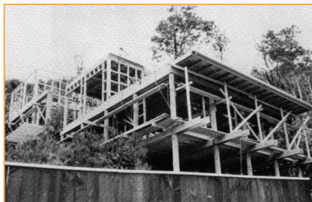
Pole structure with frame for lower level and platform for higher levels.
