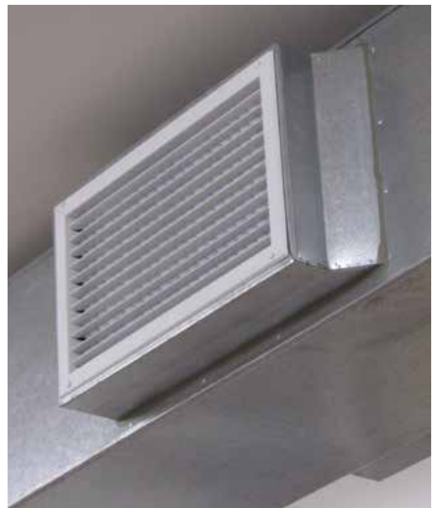
Cleaning access for ducts.
