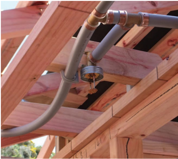
A sprinkler head directly attached to a piping loop in the ceiling of a house. The sweeping curve of the pipe [on the left] means fewer fittings are required and improves the efficiency of the flow.
