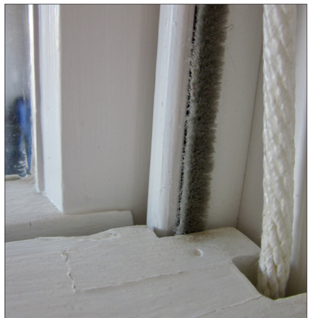
Figure 6. Brush pile seal in double-hung window.
