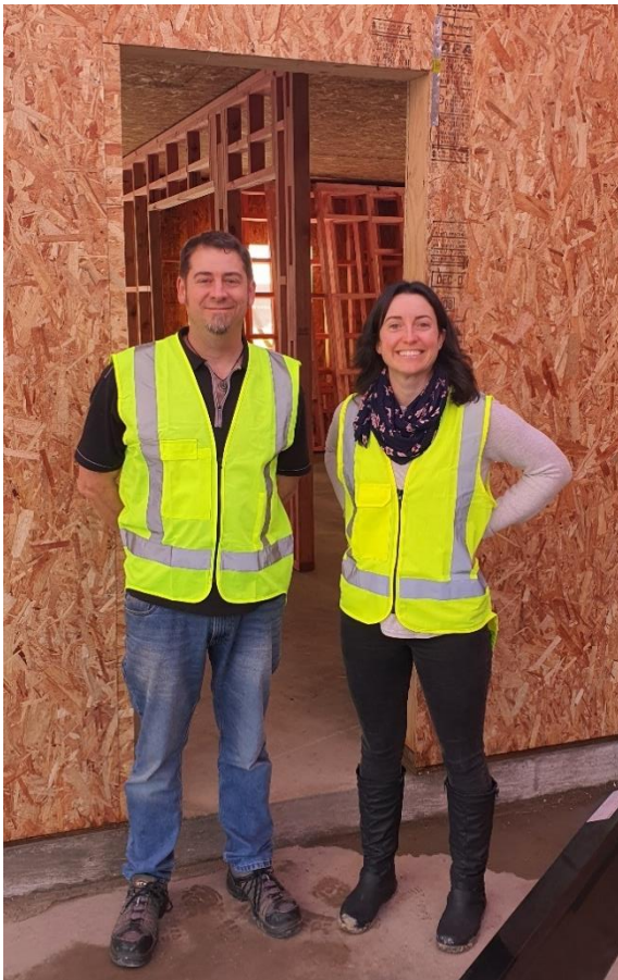
BRANZ researchers Dr David Carradine and Anna Walsh inspect a SIPs building under construction (photo credit: Nick Hubbard)
