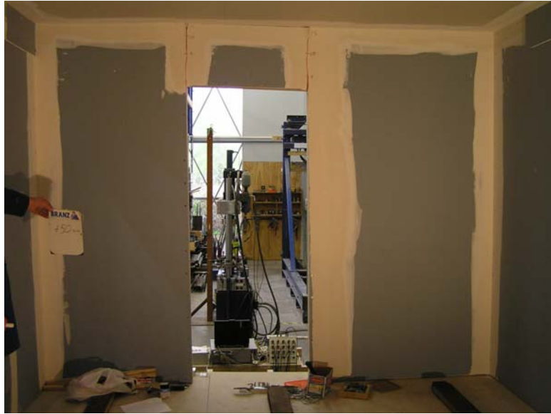
Figure 56. Plasterboard cracking at End 2 in Stage IV.
