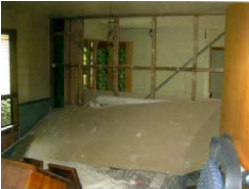
Figure 2 Failure of generic plasterboard/metal brace combination (Buchanan et al. 2011)
