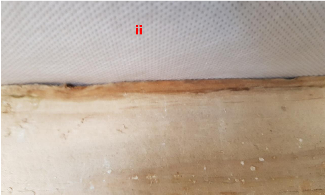
Figure A3. Close-up view of (ii) the underlay cut approximately 5 mm longer and tucked between the framing and the back of the cladding. This image was taken after the test.
