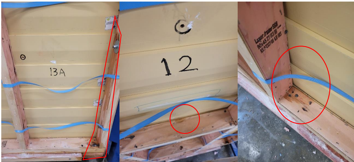
Figure 9. Close-up view – walls insulated with 20 mm separation via strapping holding the insulation and without underlay where water transfer occurred (circled).
