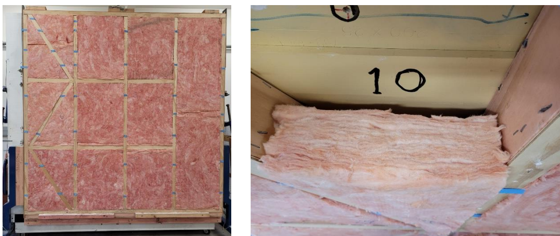
Figure 7. Walls insulated with 20 mm separation via strapping holding the insulation and without underlay.
