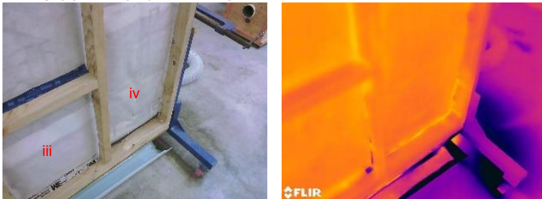
(n) (iii) Underlay taped to framing, (iv) strip of kraft paper tucked between framing and underlay
