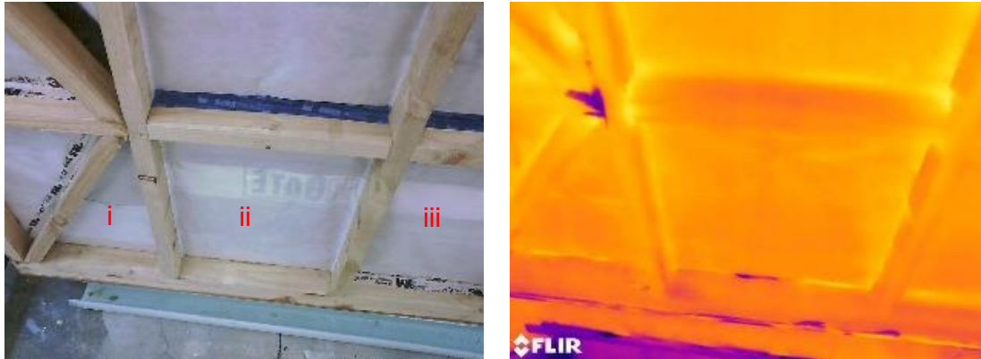
(m) (i) Underlay cut to fit the cavity, (ii) underlay tucked between bottom plate and back of cladding, (iii) underlay taped to framing
