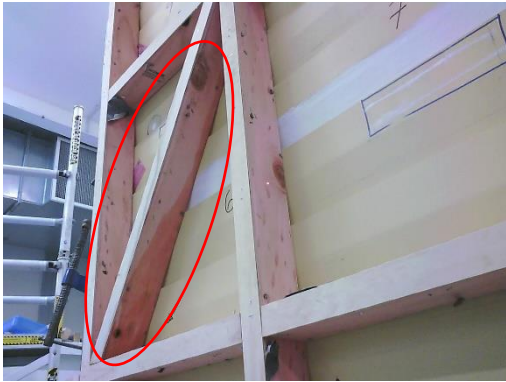
(a) Water was transferred to diagonal bracing
